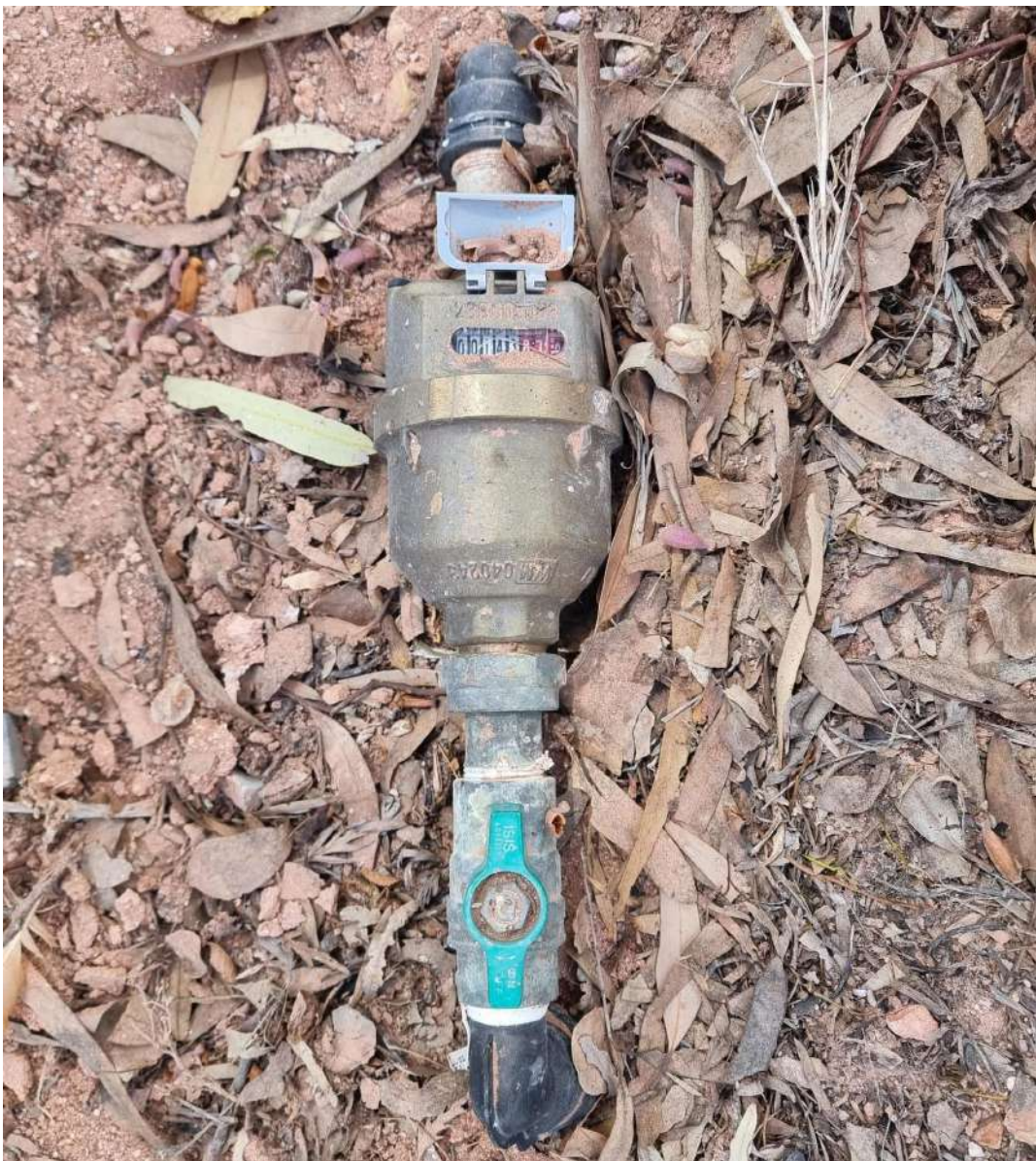
A typical Coober Pedy water metre
