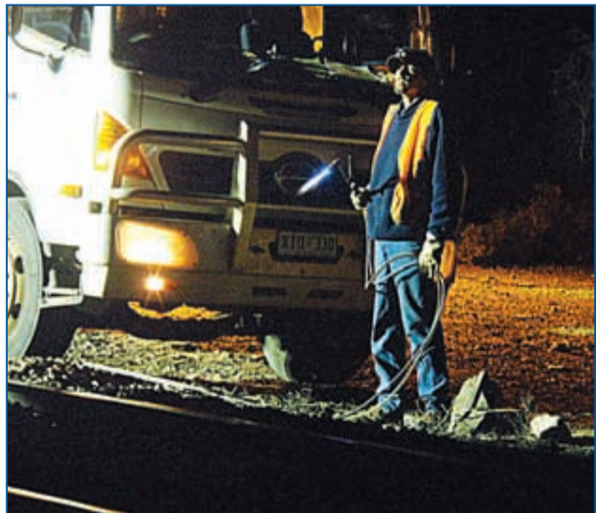
During a 12 hour ordeal, workers repaired damages and returned the train to its tracks. Photo: Nellie Malseed
